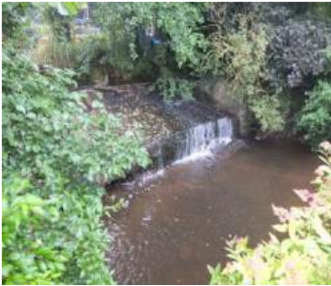
This weir on the River Wolf Acts acts as a complete barrier to fish trying to access the middle and upper river
