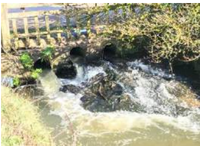
As example of Irish Bridge with water channelled through a series of fish unfriendly pipes on the R Love.
