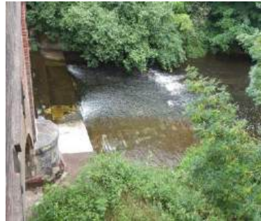
View of the apron of Fenny Bridge which acts as a partial barrier to fish
