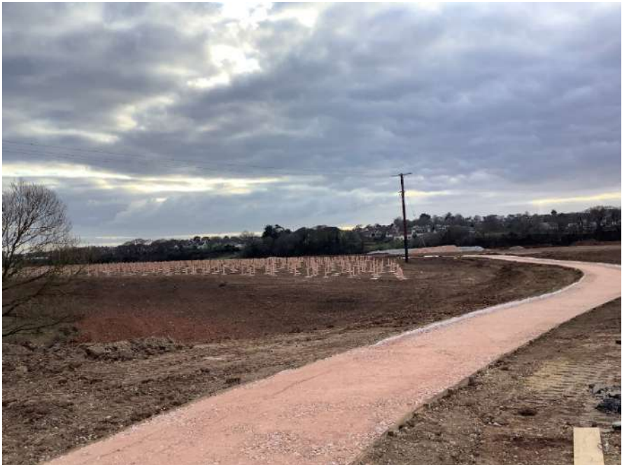
The site of the former Budleigh Tip will be enhanced by the planting of over 12,000 trees
